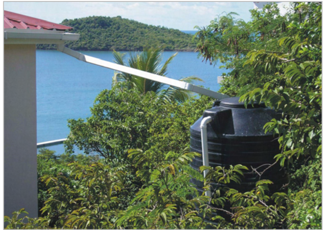
Typical household rooftop rainwater harvesting in southern Grenada (Woburn).
