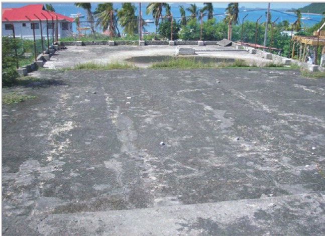
Concrete rainwater catchment surface in Petit Martinique.
