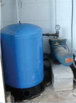
Figure 26 Pressure tank (left) and pump
