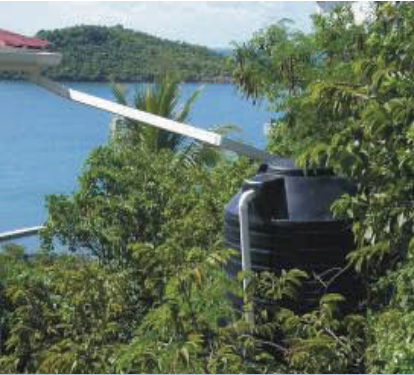
Figure 22 Typical plastic tanks for household RWH system
