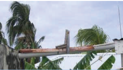
Figure 30 An example of a rat guard along a gutter to a storage tank in the Grenadines
