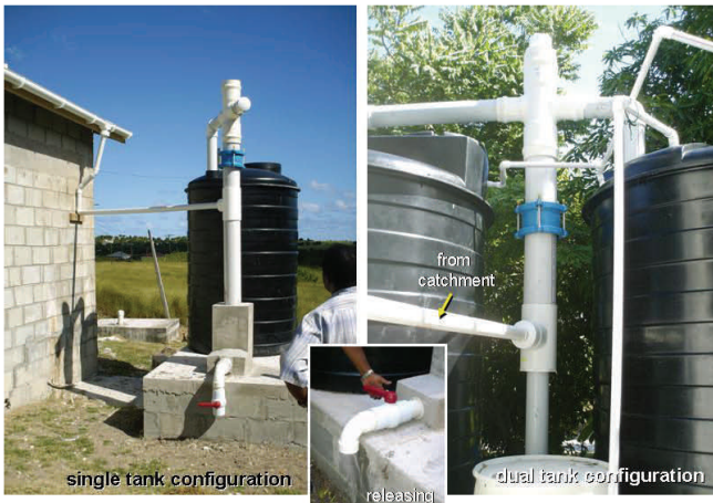
Figure 14 Examples of up-flow filter first-flush diverters (single and dual tank configurations). Used in UNEP/CEHI RWH Project Antigua and Barbuda
