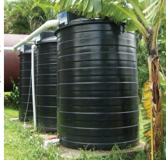
Figure 18 Multiple PVC tanks for rainwater storage
