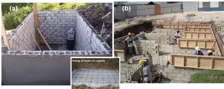
Figure 21 Typical block-type cisterns under construction (a) household (b) commercial applications (photos courtesy Dr. Everson Peters and Andrew Hutchinson)
