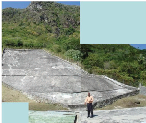
Figure 6 Surface catchment for communal RWH system at Ashton on Union Island, St. Vincent and the Grenadines
