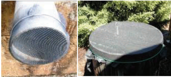
Tank overflow covered with fine mesh
