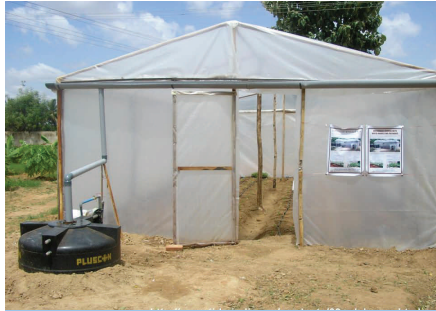
Figure 34 Rainwater harvesting off a greenhouse for irrigation purpose Source: Technology Informatics Design Endeavour (TIDE) http://www.tide-india.org/products/06polyhouse.html
