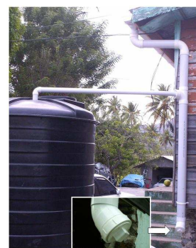
First-flush diverter and storage
