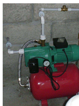
Pump and pressure tank
